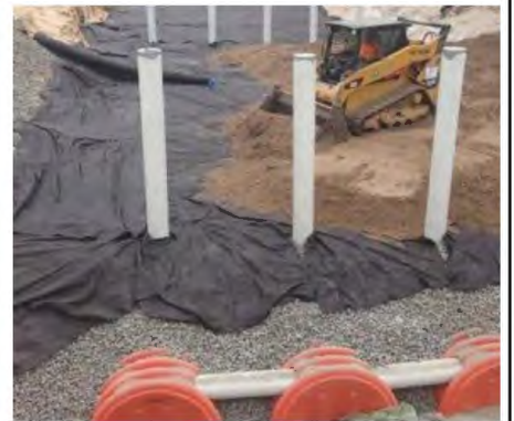
PVC Cleanouts (vertical) Flow Connection Pipes (horizontal)
