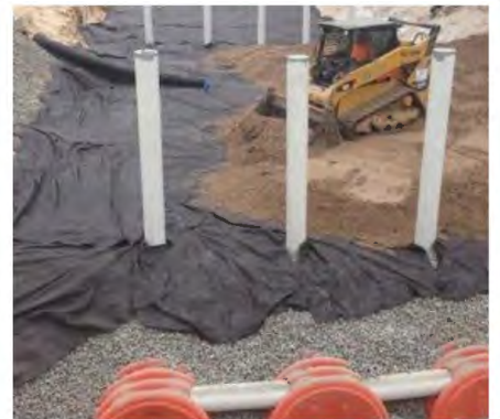
PVC Cleanouts (vertical) Flow Connection Pipes (horizontal)
