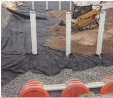
PVC Cleanouts (vertical) Flow Connection Pipes (horizontal)
