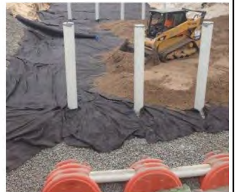
PVC Cleanouts (vertical) Flow Connection Pipes (horizontal)
