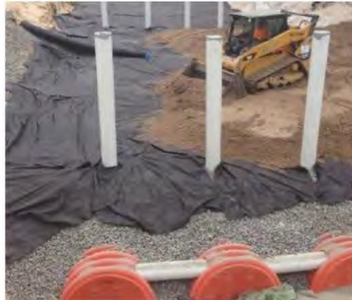
PVC Cleanouts (vertical) Flow Connection Pipes (horizontal)
